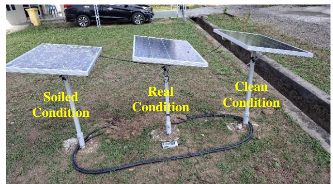
Fig. 3. Experiment PV Module Installation Outdoor.
